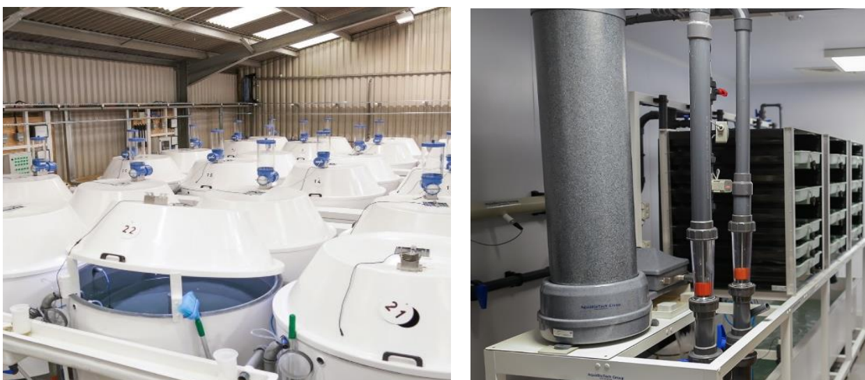
Fig. 3. Facilities available at the Niall Bromage Freshwater Research Unit located at Buckieburn, Institute of Aquaculture.
